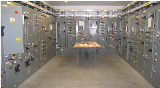
View of the new electric control cabinets at pit.
