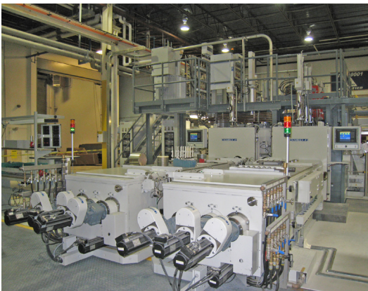
View of the new electric beam coater chambers.
